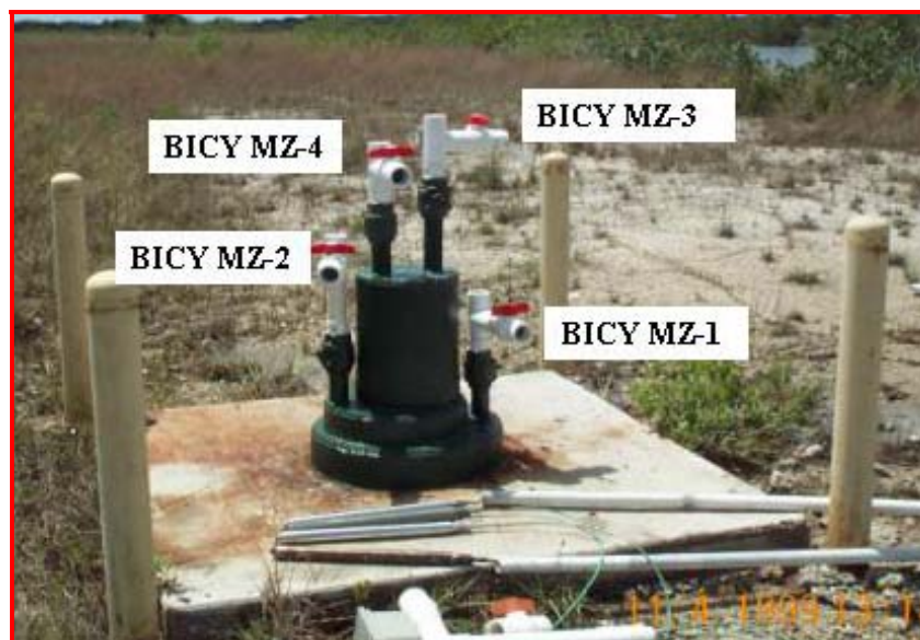
Figure 4. Photograph of Completed Test Monitor Wellhead (BICY-TW).
