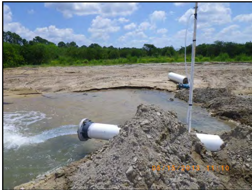
FIGURE 15: PUMP TEST SET-UP
