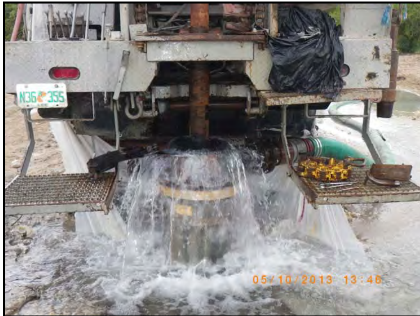
FIGURE 11: FREE FLOW AFTER DEVELOPMENT AIR DEVELOPMENT
