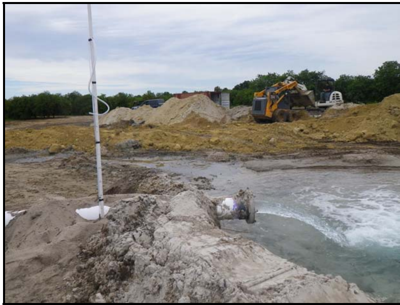
FIGURE 17: PUMP TEST SET-UP
