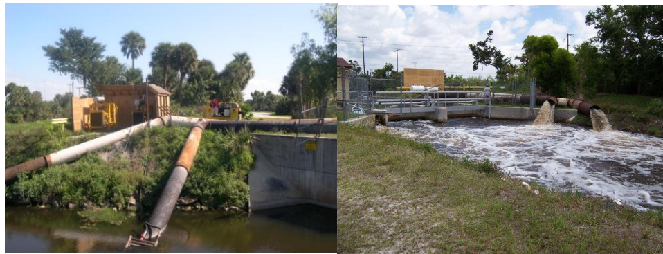
Figure 3. Temporary pump installation at Control No. 2 site: Left) Intake side; and Right) Discharge end.
