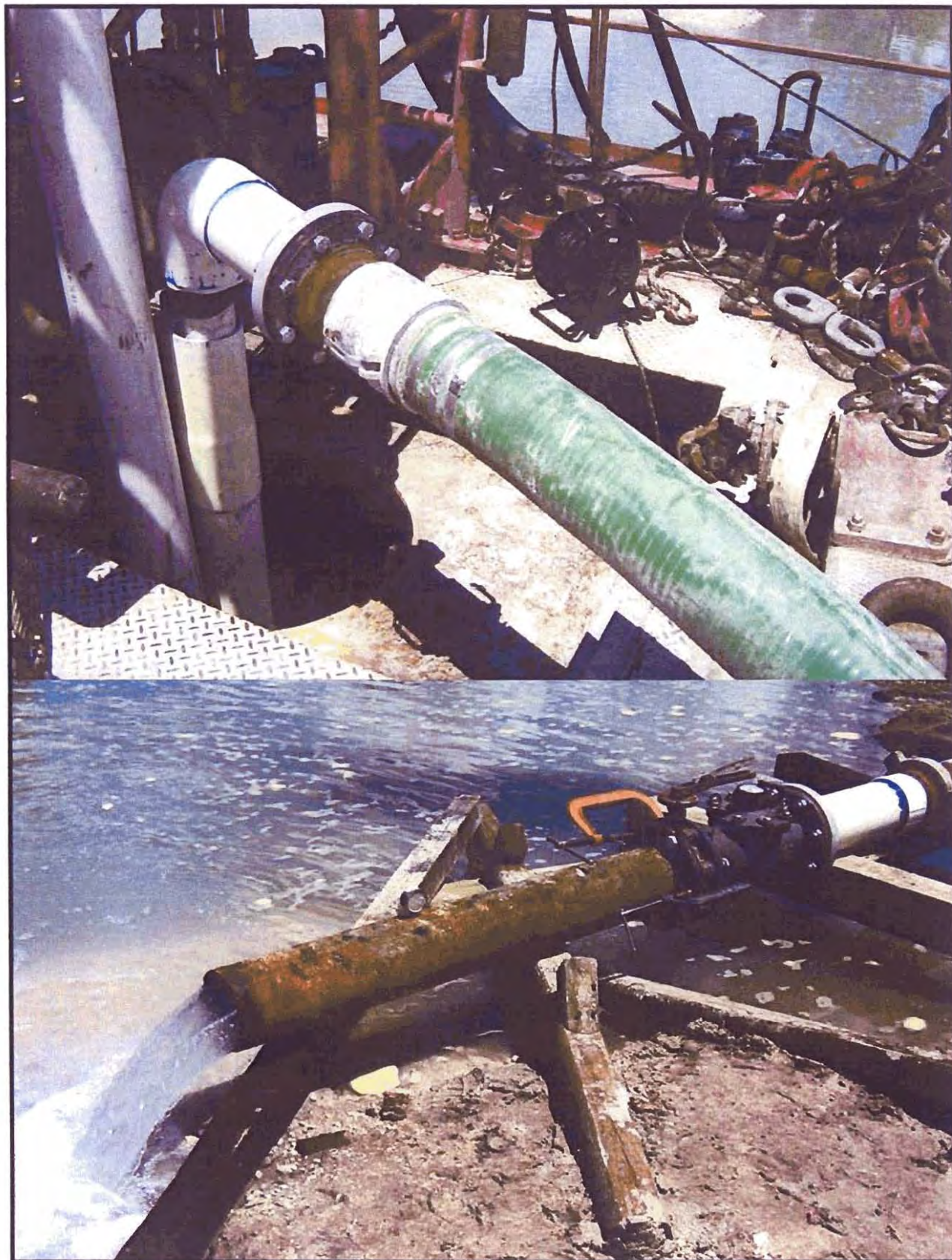
Figure 27 – Step Testing Drop Pipe and Discharge Assembly
