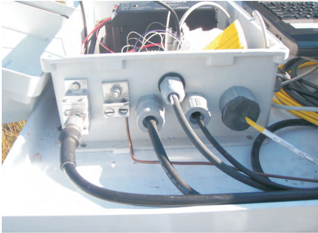
End view of instrument enclosure housing datalogger and battery at MW-5 11 Oct 2010.
