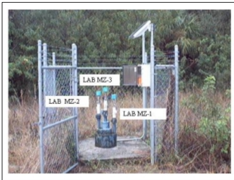
Figure 4. Photograph of Completed Tri-Zone Monitor Wellhead and Fence Enclosure (LAB-TW).
