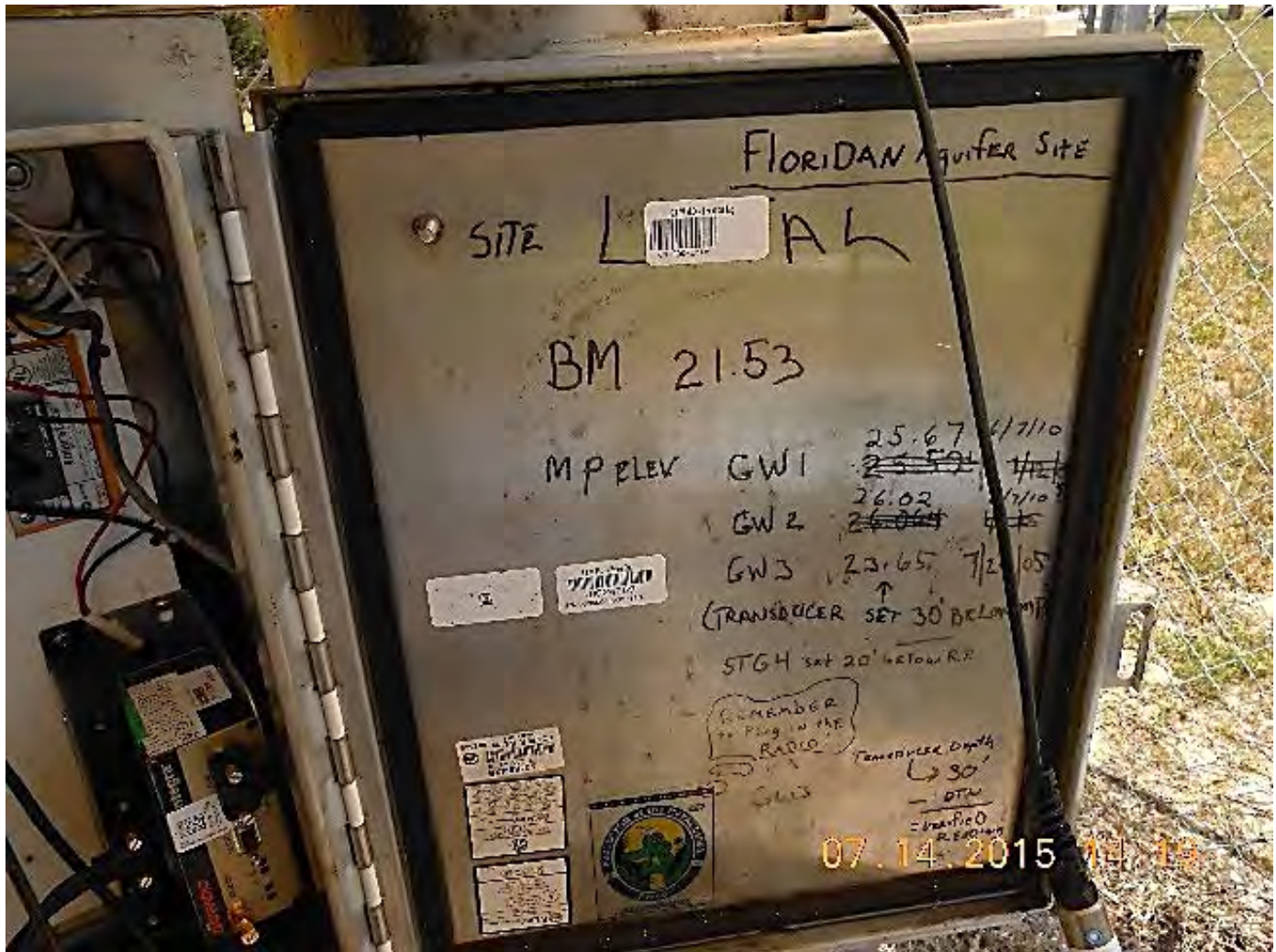
RTU Inside Panel
