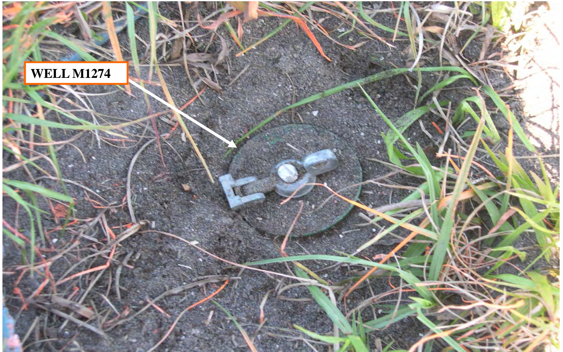
Biscayne Engineering Company, Inc. Date of Photo: 01-15-06 View: Well M-1274
