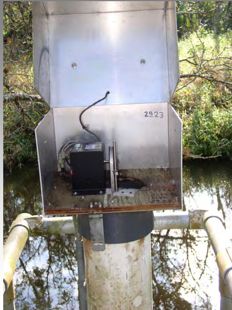
South Florida Water Management District Date of Photo: February 3, 2005 View: Looking easterly at open recorder box
