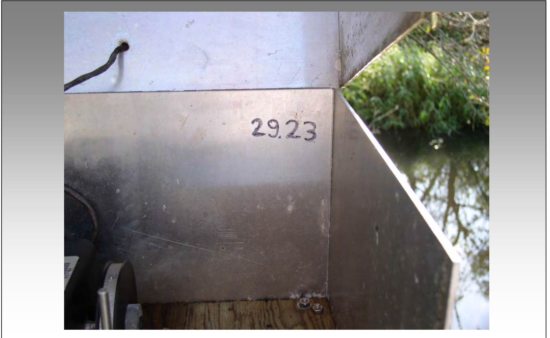
South Florida Water Management District Date of Photo: February 3, 2005 View: Looking easterly at the Recorder Box
