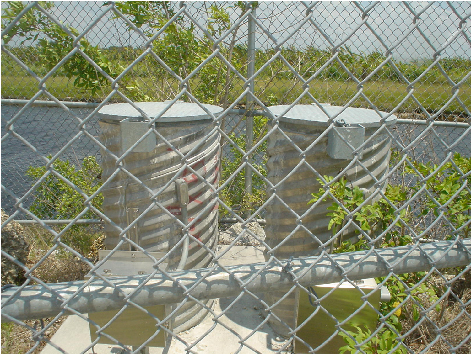
Weidener Surveying & Mapping, P.A. Date of Photo: April 26, 2005 View: Monitoring Wells 1A and 1B
