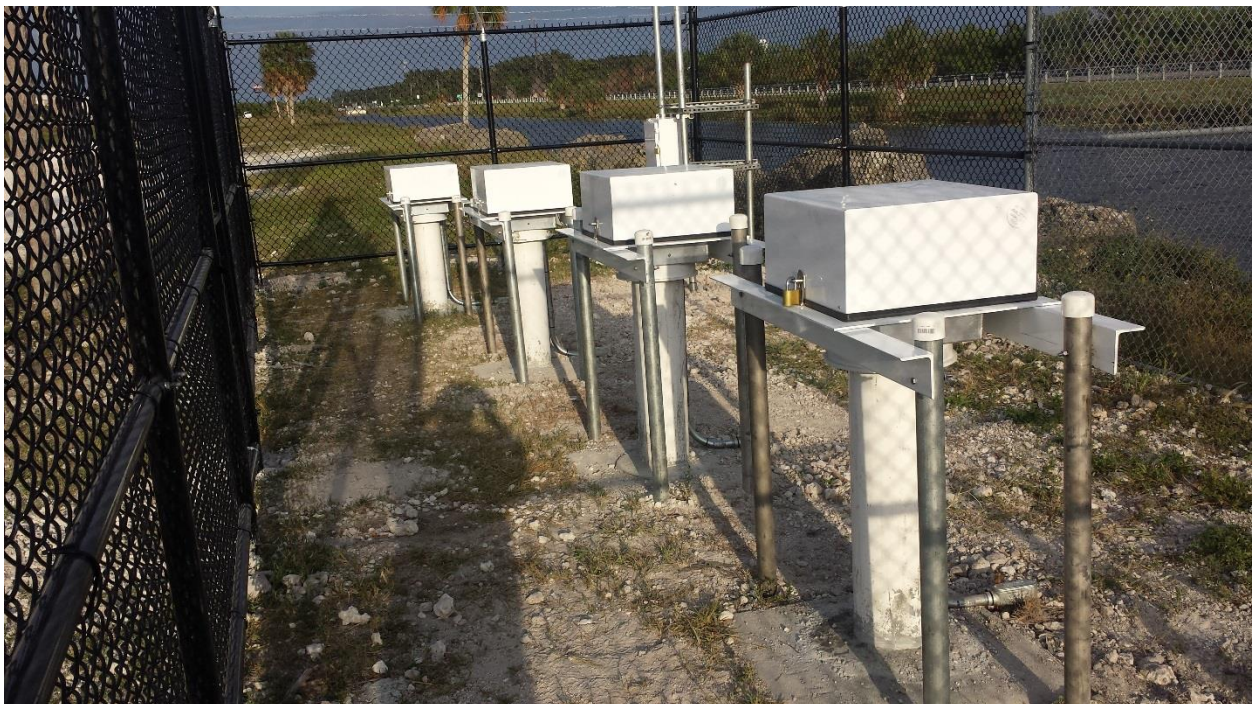
Figure 8. S-356 well heads equipped with service platforms and telemetry, close-up.
