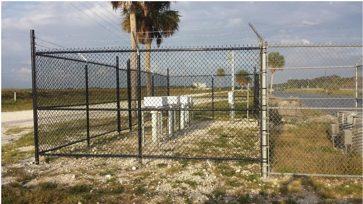
Figure 7. S-356 Well heads installed with service platforms and telemetry, looking east.
