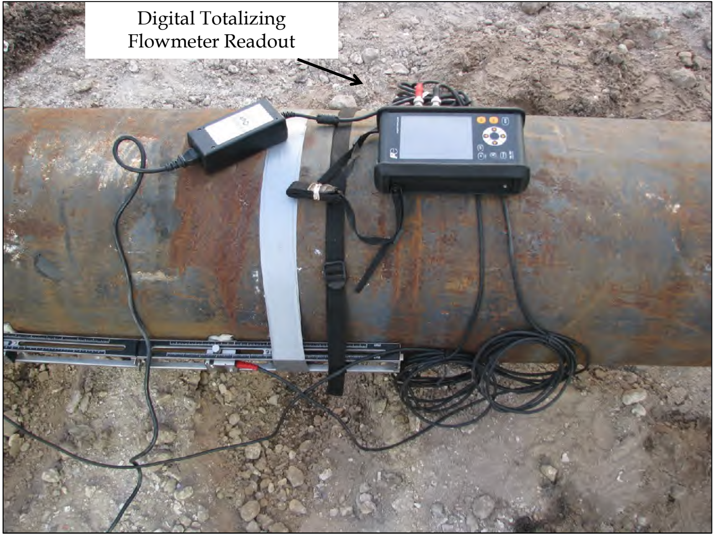
FIGURE 3-35 Strap-on Sonic Flowmeter
