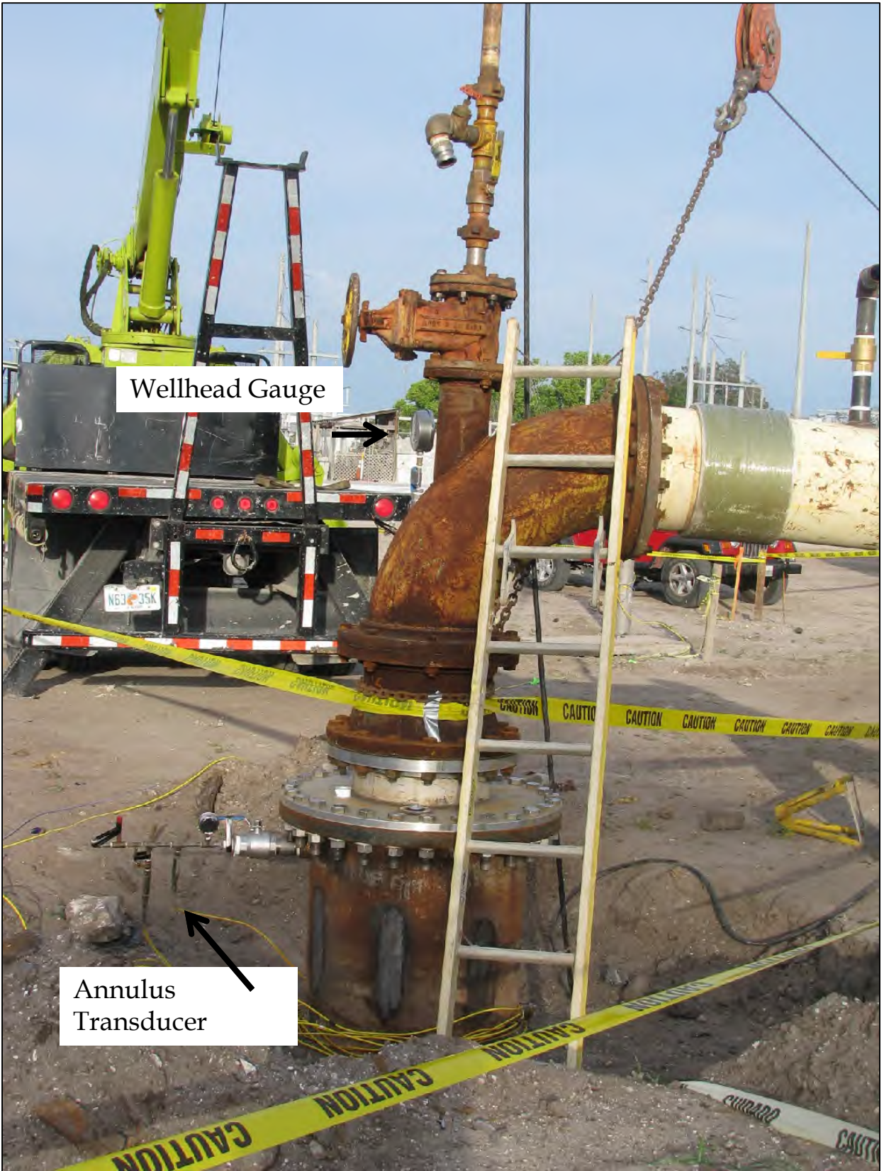
FIGURE 3-33 Injection Test Well head
