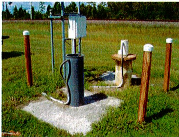
Sensor Well Area:
