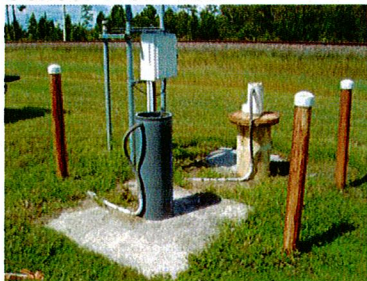
Sensor Well Area:
