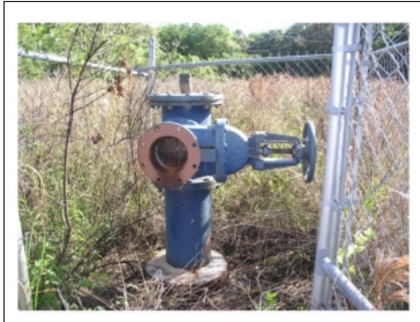
Figure 6. Photograph of Completed Test-Production Wellhead and Fence Enclosure (LAB-PW).
