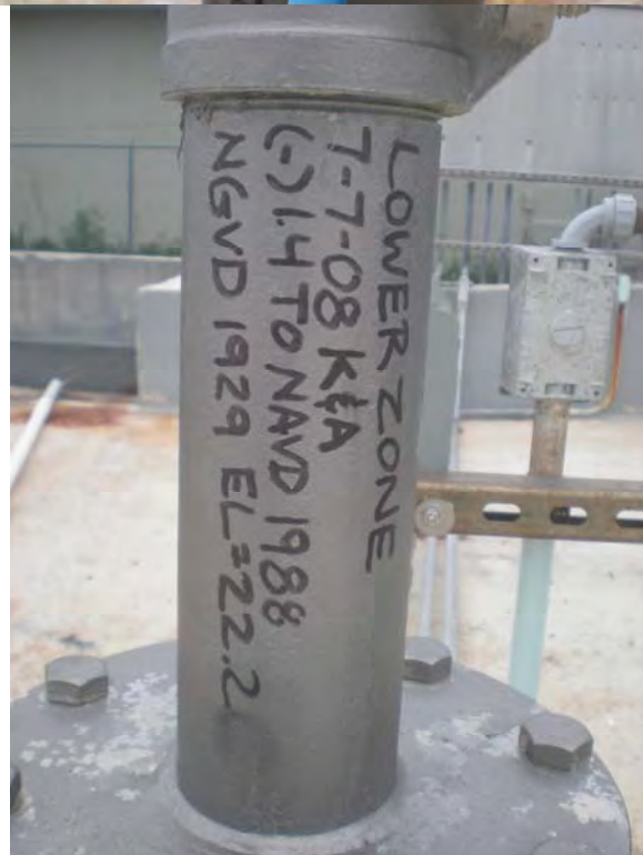
Lower Zone Well Measure Point and Information 7/07/08 Keith and Associates
