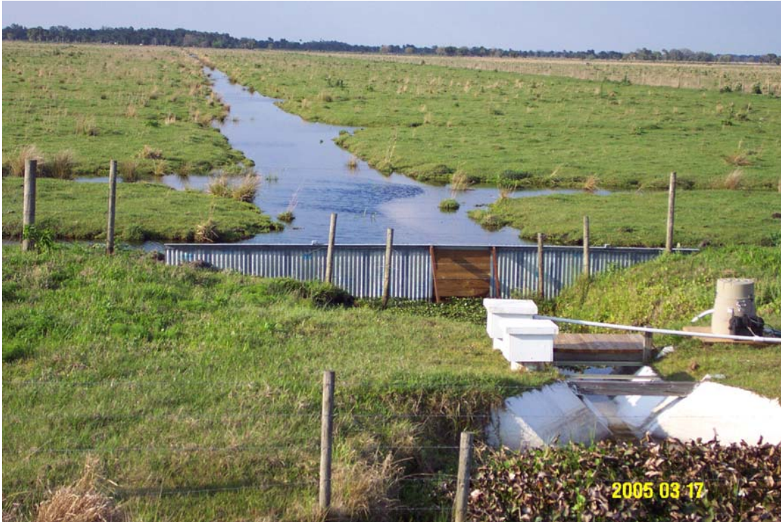
Figure 6. Photo of water control structure installed just upstream of the water monitoring station at the south end of pasture SP2. The corrugated steel structure has gap on the middle with c-channel to allow addition of wooden boards to retain water at a desired level behind the structure. Steel braces on the downstream side of the opening provide extra support at the center of the structure.
