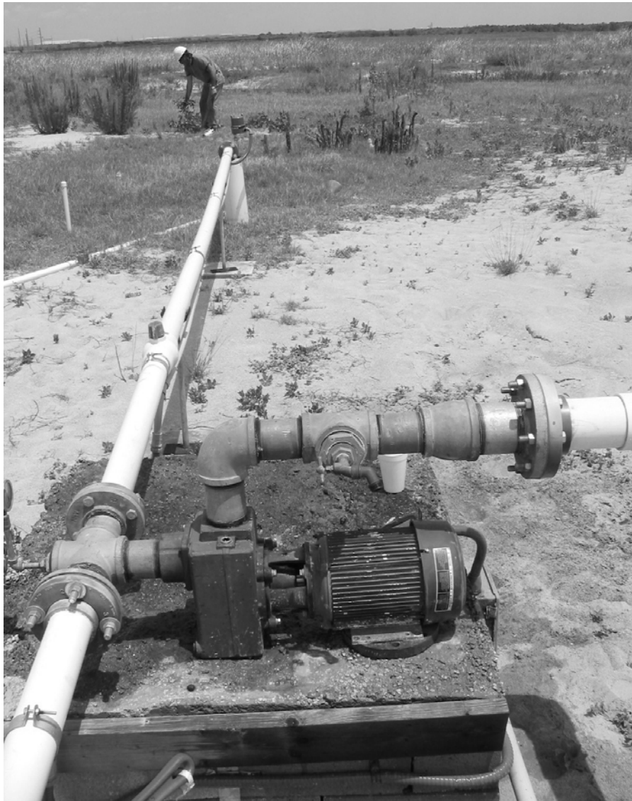
Figure C-1. Tailing Sand Filter Basin Pumping Station.
