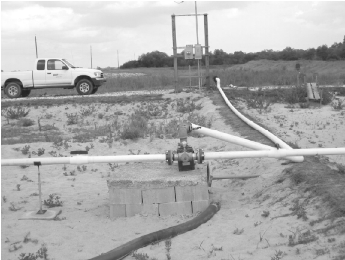
Figure C-2. Filter Basin Looking East Showing Electric Equipment.
