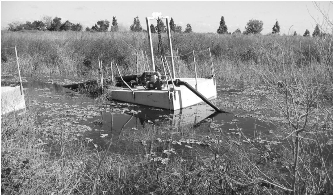
Figure C-7. Plant Island Stormwater Drainage Ditch Pumping Station.
