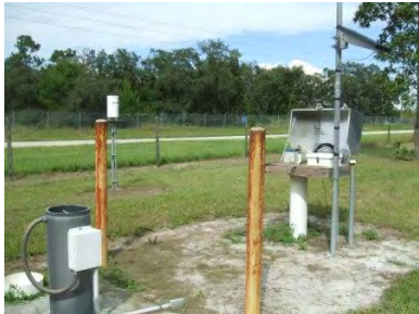
Sensor Well Area:
