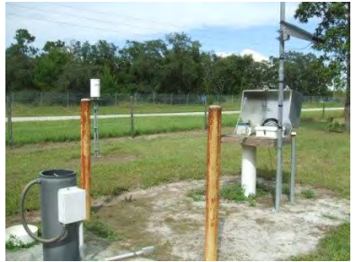
Sensor Well Area:
