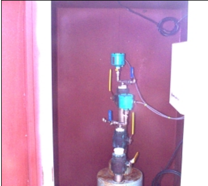
Figure 8. DF-3,4,5 Tri-Zone Wellhead.
