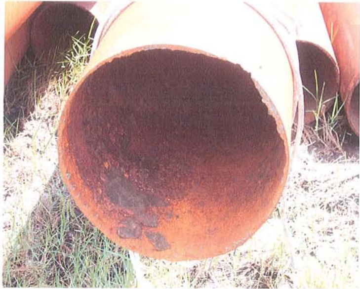
Visible thinning of the steel tubing wall removed from IW-1
