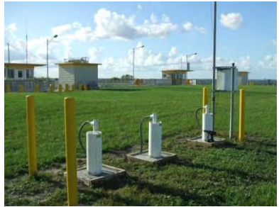
Sensor Well Area:
