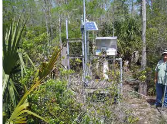
STG2 AREA LOOKING NORTH
