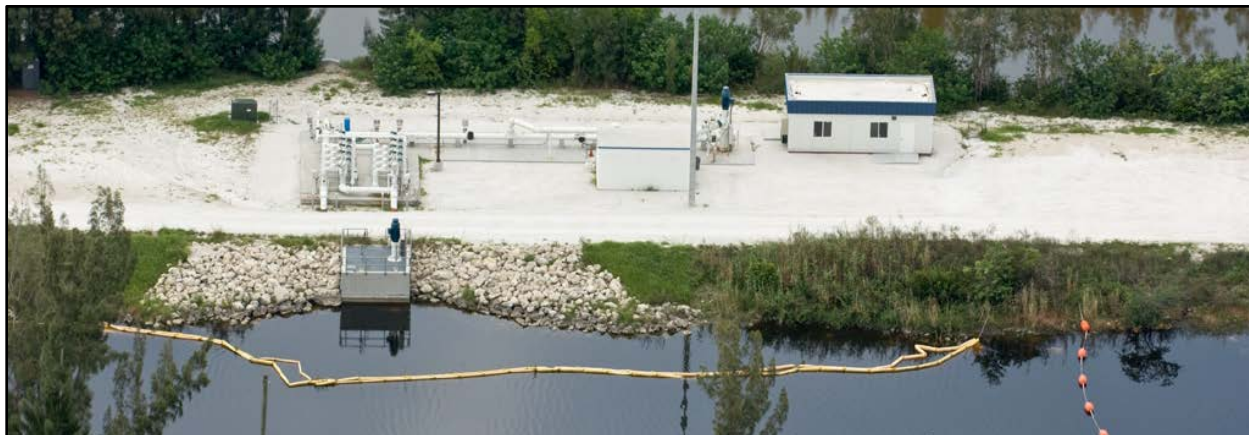
Figure 6-20 -- Aerial photograph showing the surface facility at HASR.
