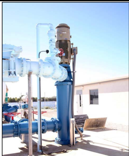
Figure 6-17 -- ASR well recovery pump.
