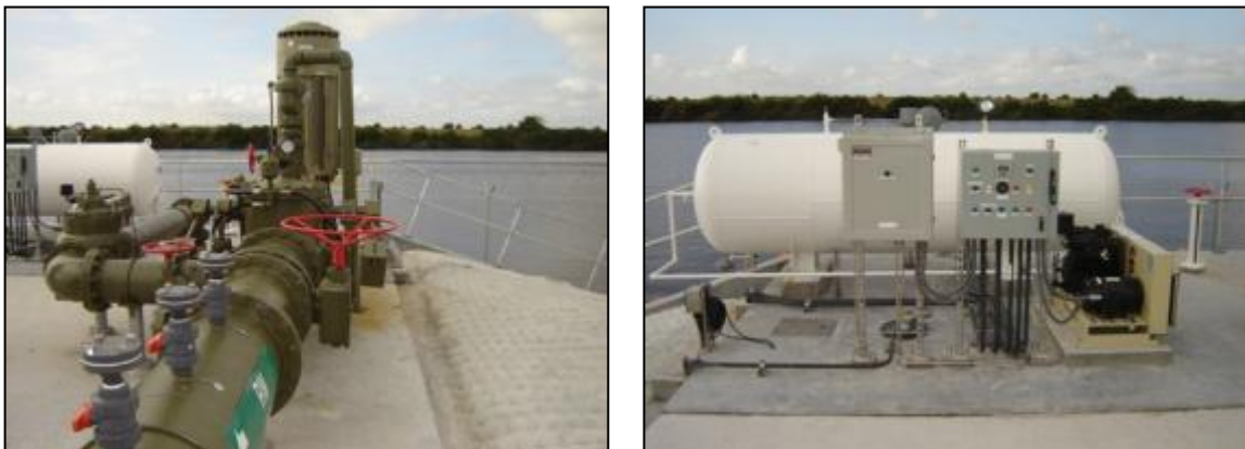
Figure 6-3 -- Recharge pump at intake (left) and air compressor (right).
