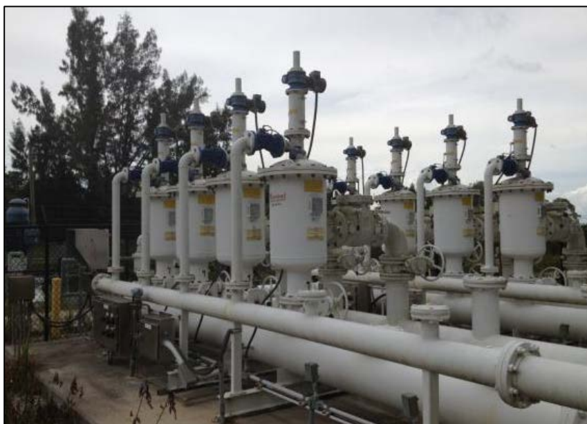
Figure 6-15 -- Amiad filtration system.
