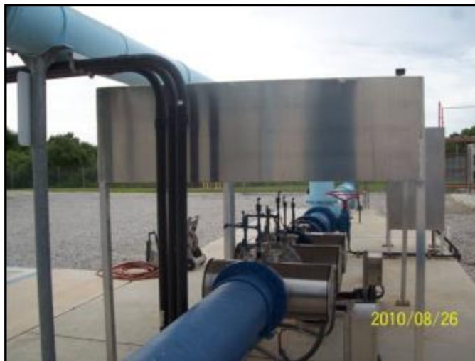
Figure 12-1 -- The UV disinfection system enclosure.
