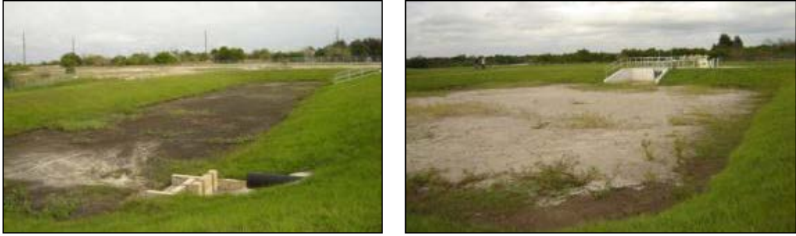
Figure 6-8 -- The backwash equalization pond (left), and solids storage pond (right).
