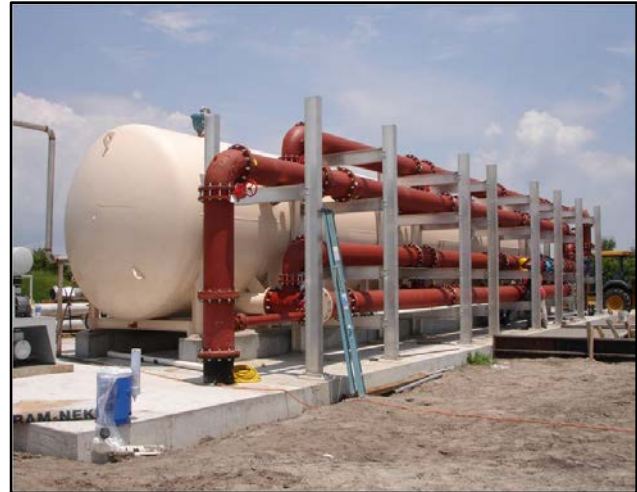
D. Influent and effluent pipes on pressure filter.
