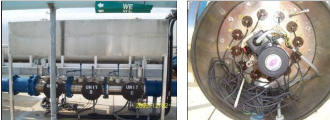
Figure 6-6 -- The UV disinfection units. Units are arranged in series (left), and a cross-section view of a single unit showing 12 UV lamps oriented perpendicular to flow direction (right).
