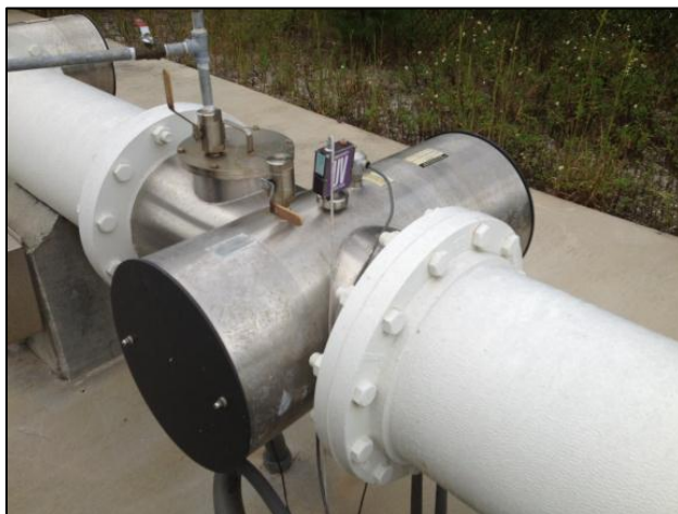
Figure 6-16 -- A single chamber of the UV disinfection unit.
