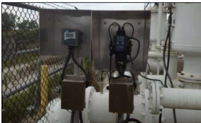
Figure 6-19 -- Water quality monitoring components.
