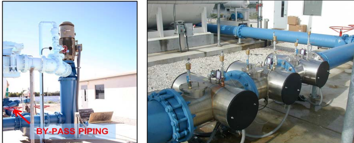
Figure 8-6 -- Completed by-pass piping (left), completion of 3-unit, in-line UV disinfection system (right).
