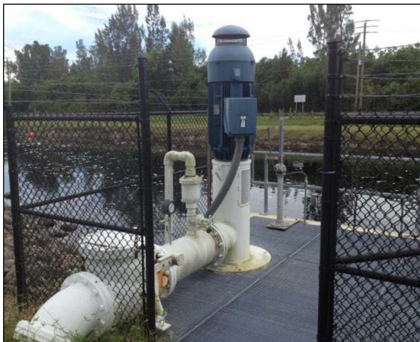
Figure 6-14 -- Recharge pump at the intake structure.
