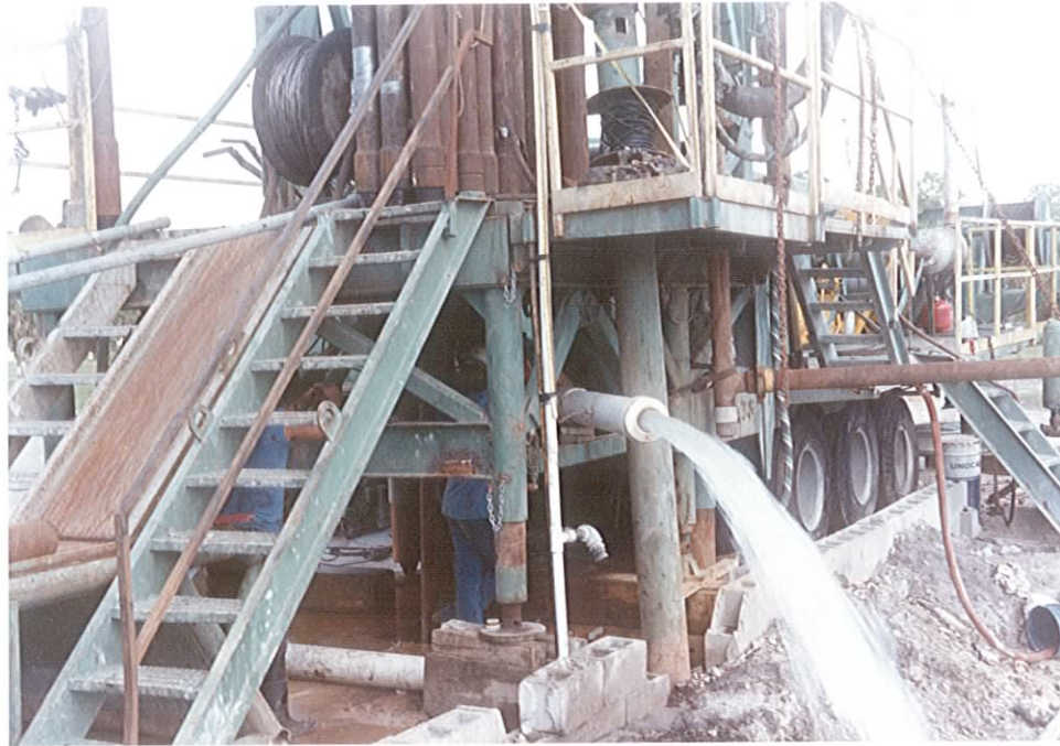
PHOTO 3. Measurement of flow quantity by use of orifice weir, CO-2080
