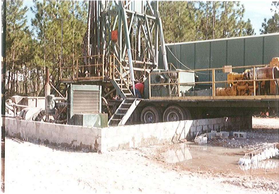
PHOTO 1. Drill rig work area surrounded by concrete block wall for water control CO-2081
