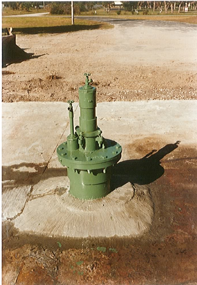
PHOTO 4. Dual completion well head, CO-2080
