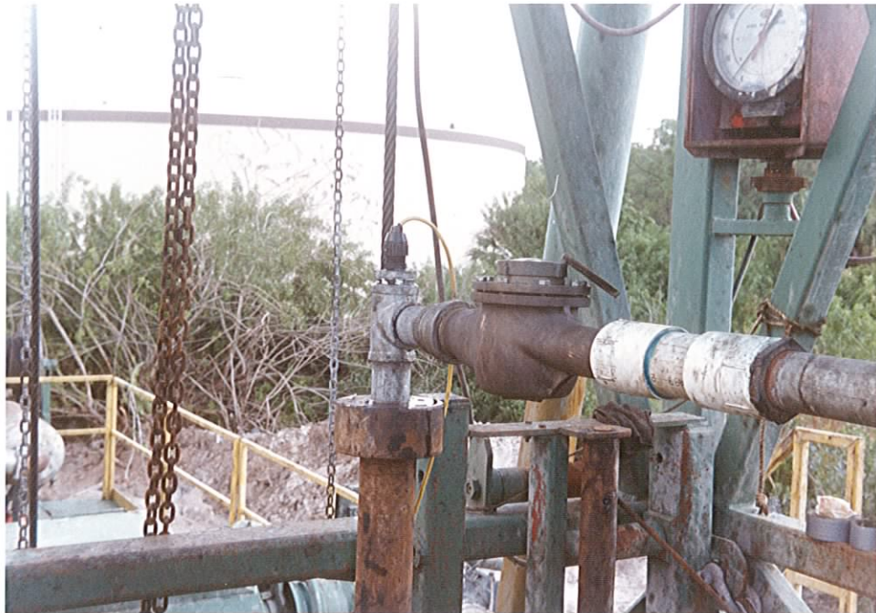
PHOTO 2. Packer flow test with pressure transducer cable and flow meter showing CO-2080
