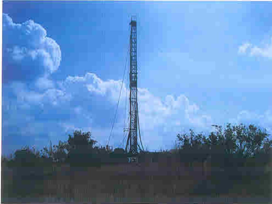
Photograph D-1- Gardner-Denver 3000 trailer mounted drill onsite at Holly Hill LFA Exploratory Well Drill Site.
