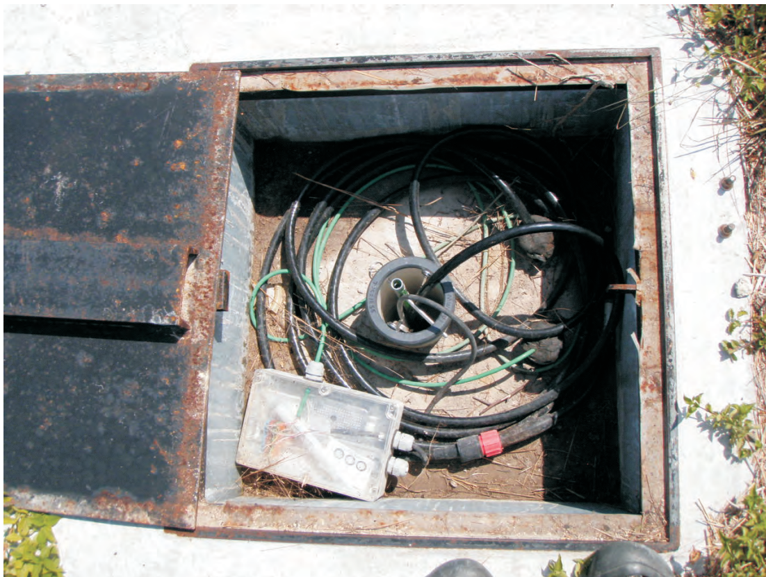
MW-1 well vault prior to cleanout of debris. 10 May 2011 The pressure transducer and flowmeter cables are suspended from the gray PVC collar using a woven wire cord grip
