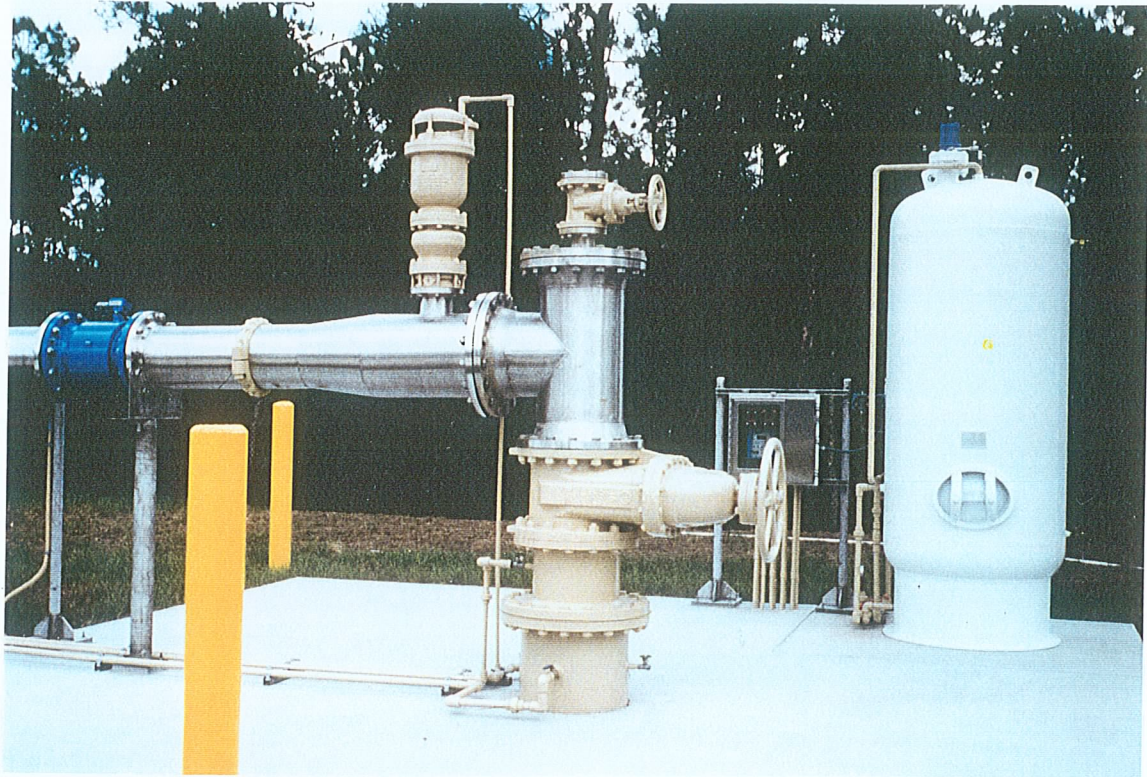
WELLHEAD AND HYDROPNEUMATIC TANK
