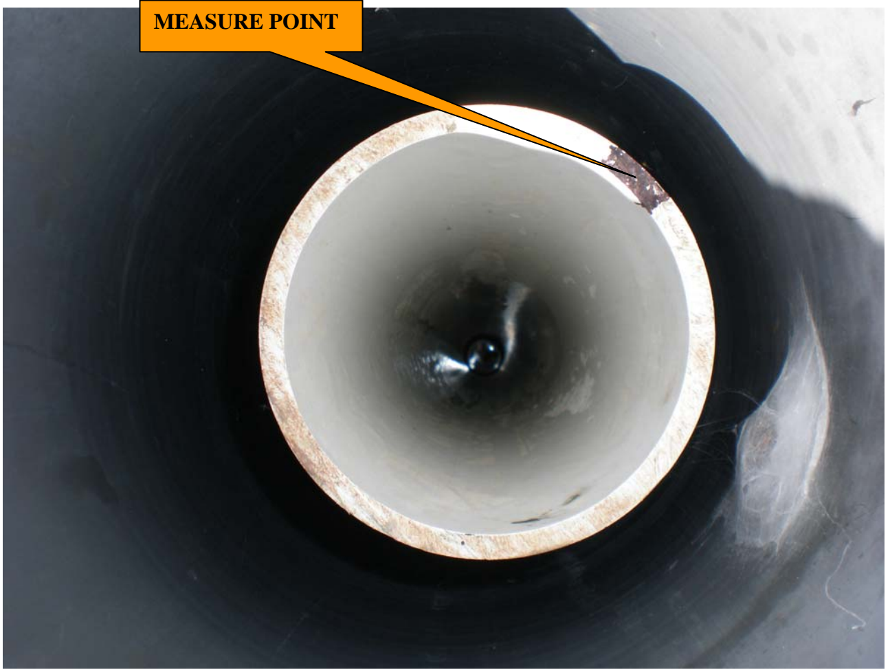
Well POS 6 Measuring Point
