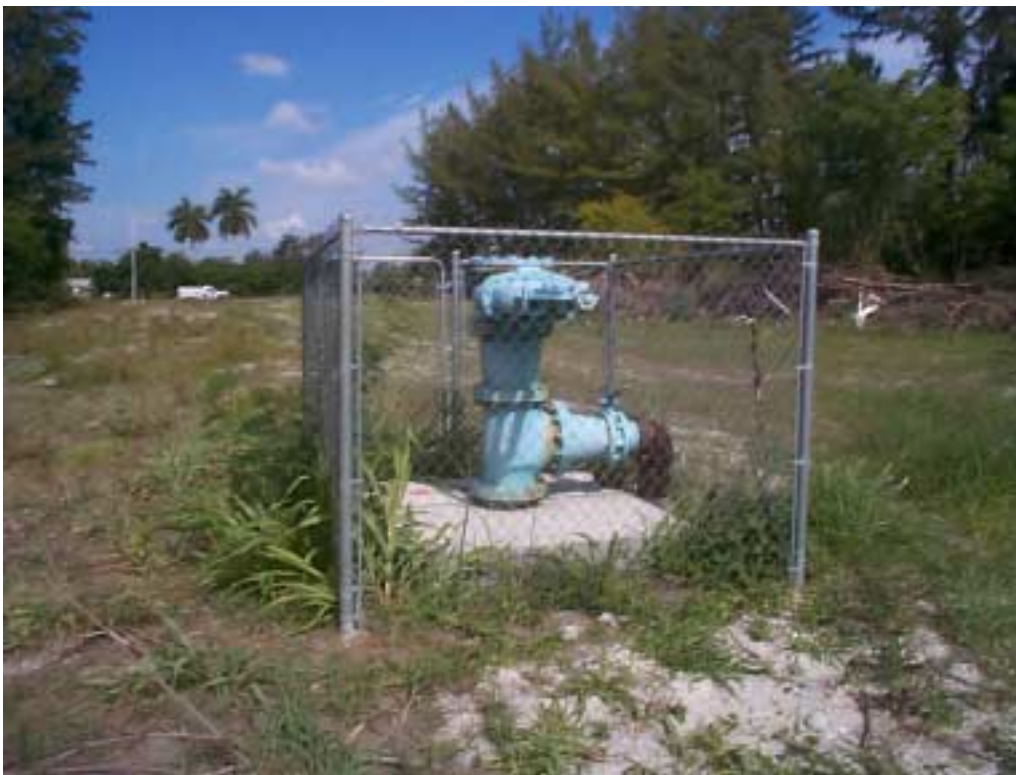
Figure 5. Well PBF-6 Completed Wellhead.
