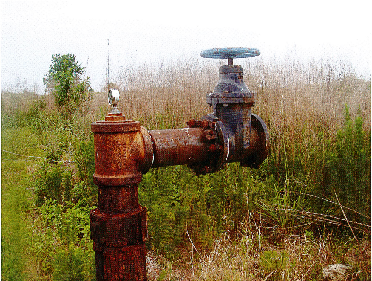
Current photograph of the artesian well located on the subject property.
