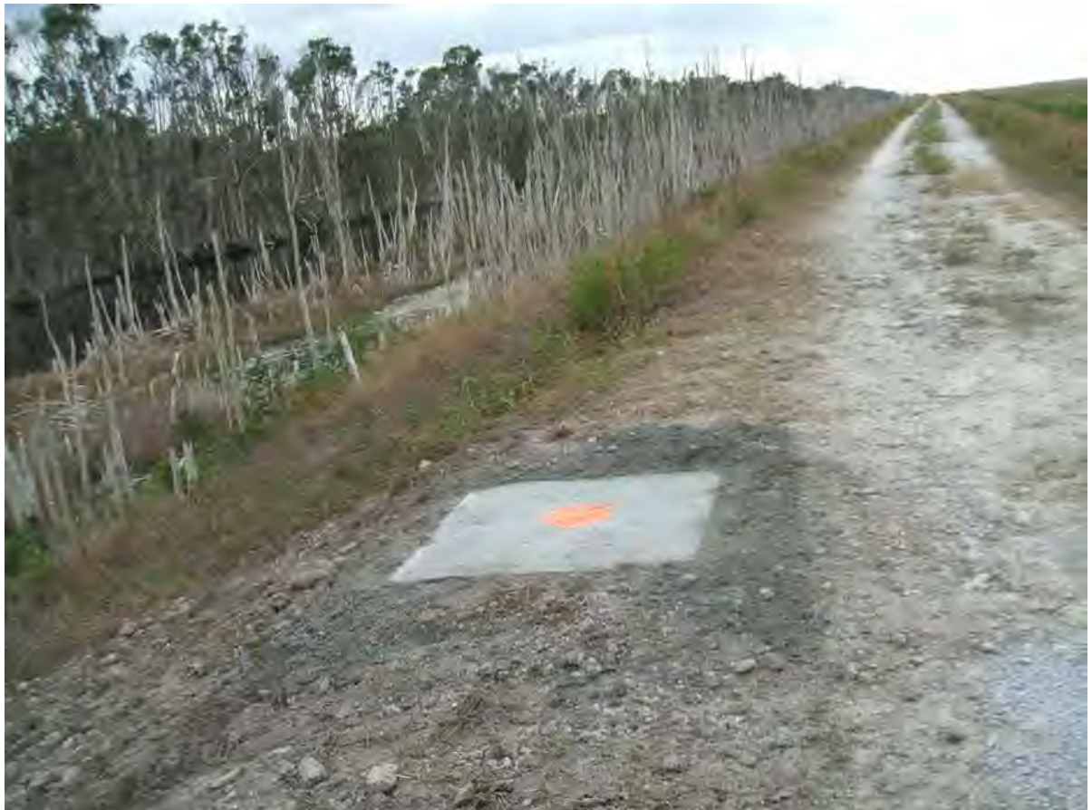
COMPLETED FLUSH MOUNT WELL PAD ON SOUTHSIDE OF L-30 WITH BOLTDOWN MANHOLE COVER
