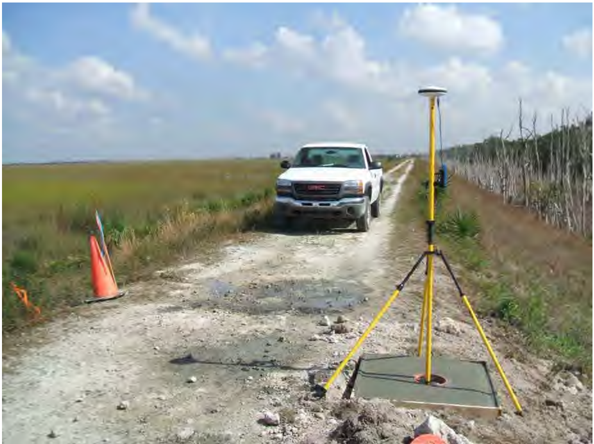
FLUSH MOUNT MONITORING WELL PADS CONSTRUCTED ON TOP OF L-30. GPS POSITIONING CONDUCTED ON WELL CASING
