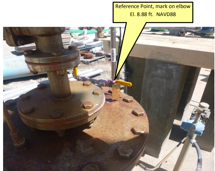
MIUGW Well Close up
