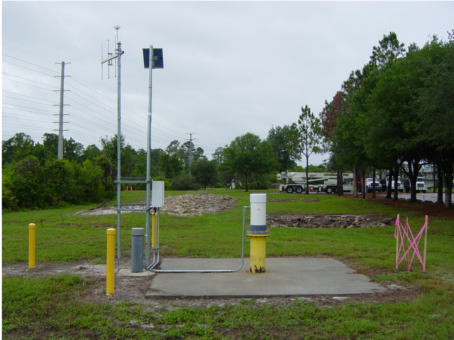
Nick Miller, Inc. Date of Photo: June 12, 2006 View: Looking at the well REDYCK facing south
