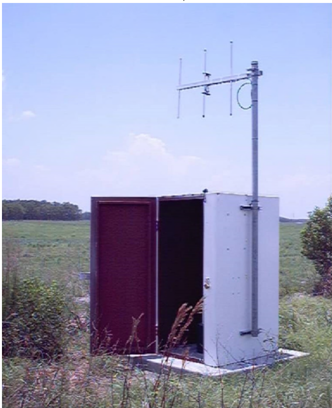
Photo 4 : OSF-62, showing antenna.
