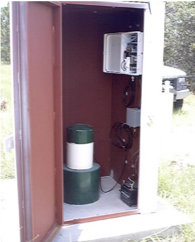
Photo 2: OSF-62 fully instrumented, view from the south.
