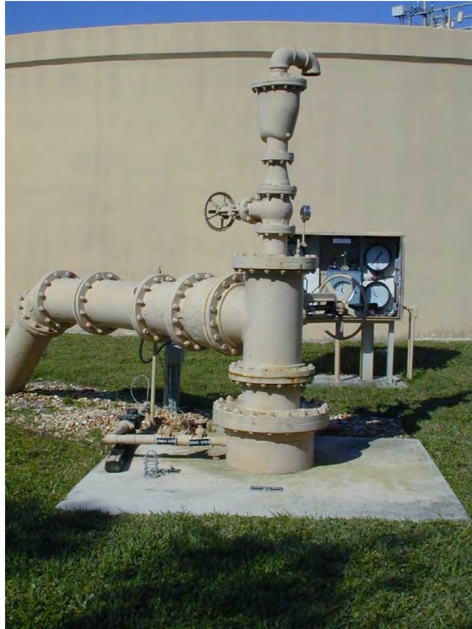
Nick Miller, Inc. Date of Photo: January 18, 2005 View: Looking at the injection well #1 facing north
