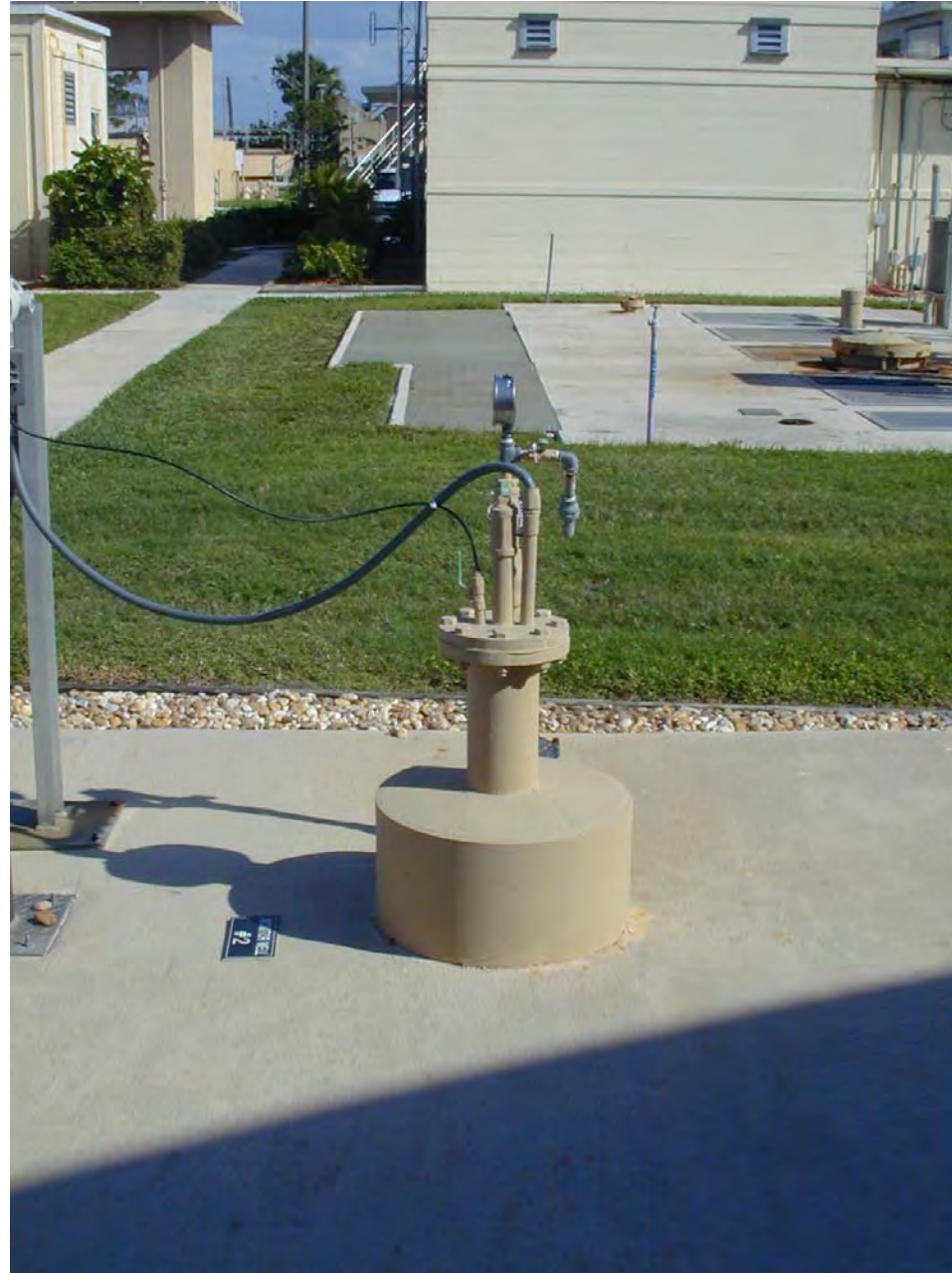
Nick Miller, Inc. Date of Photo: January 18, 2005 View: Looking at the monitoring well #2 facing east
