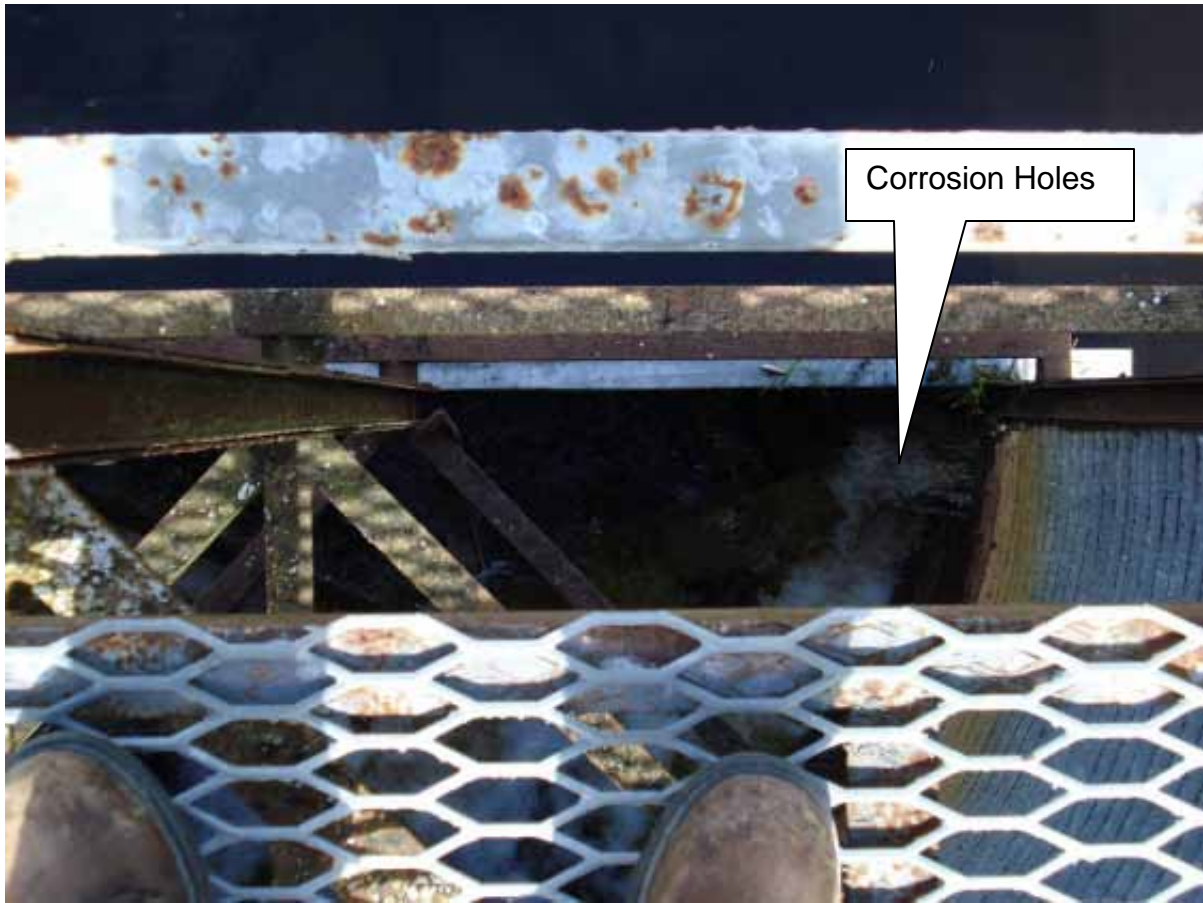
Figure 4.2.38 – Photograph of Corrosion at G-136
