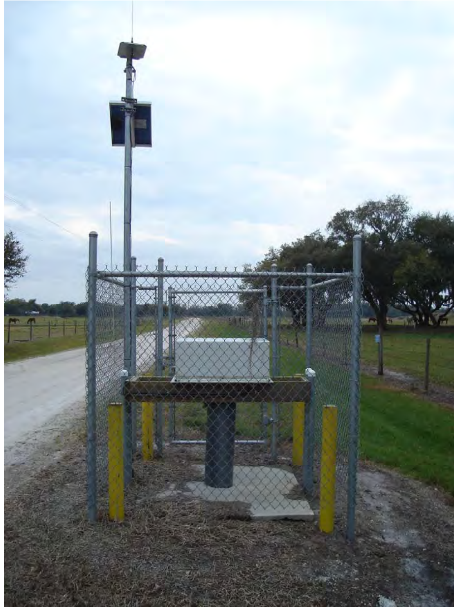
Nick Miller, Inc. Date of Photo: February 15, 2007 View: Looking at the well facing south
