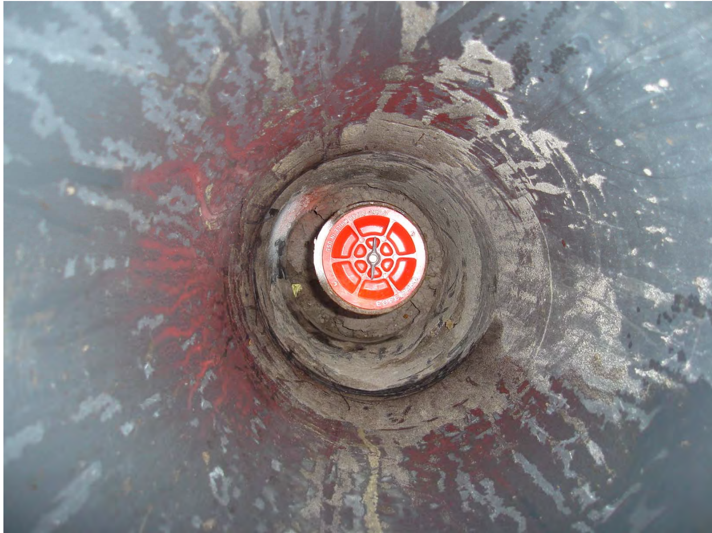
Nick Miller, Inc. Date of Photo: February 15, 2007 View: Close-up of the showing the contractor's markings on well south of well LKBA2B
