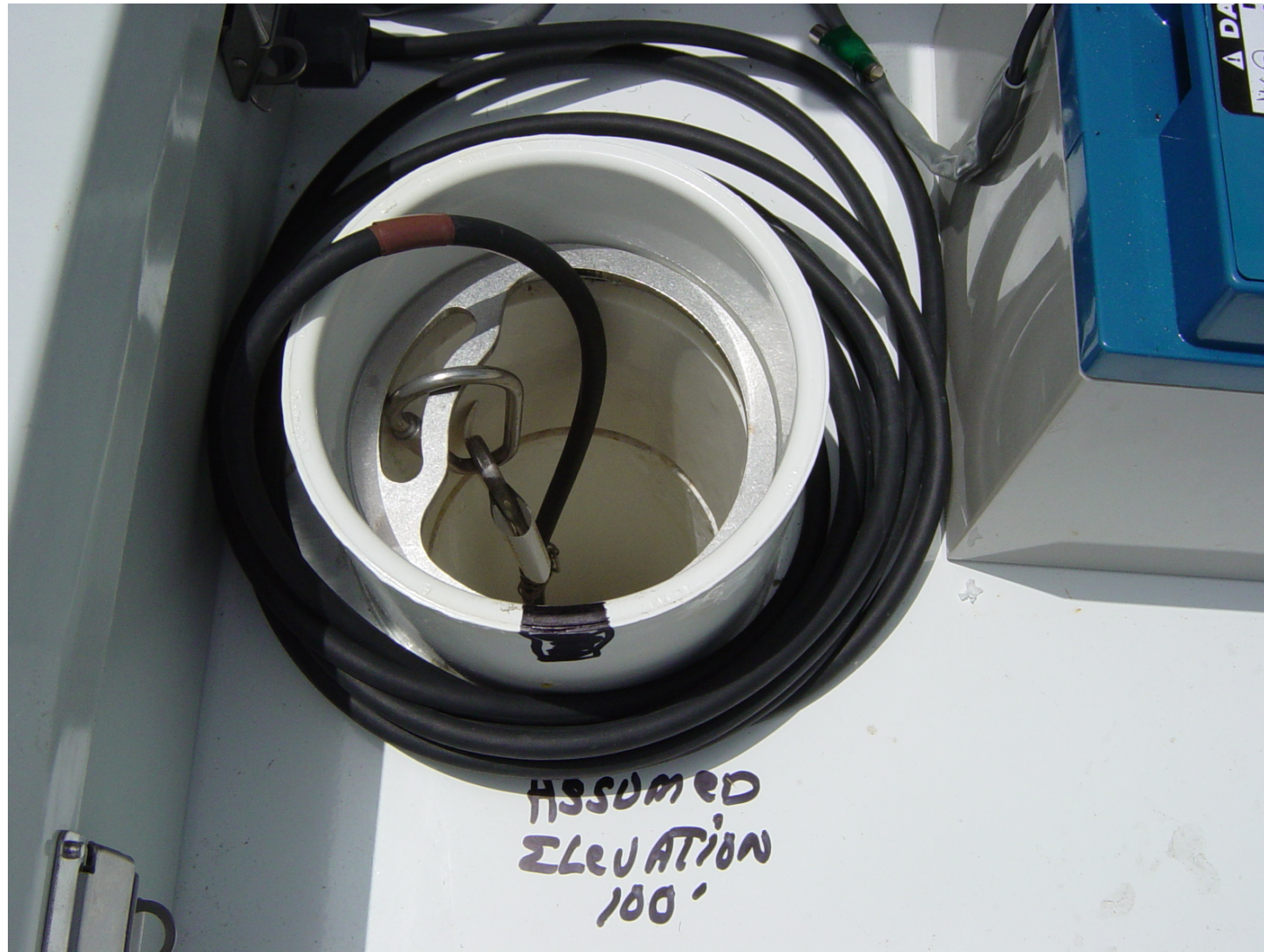
Nick Miller, Inc. Date of Photo: July 31, 2006 View: Close-up of the well showing the contractor's markings
