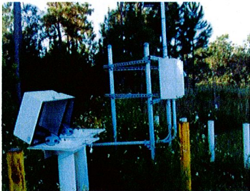
Sensor Well Area:
