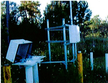
Sensor Well Area:
