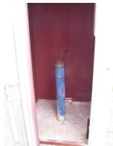
Photograph 1: BF-1 (Lower Floridan Aquifer Well)
