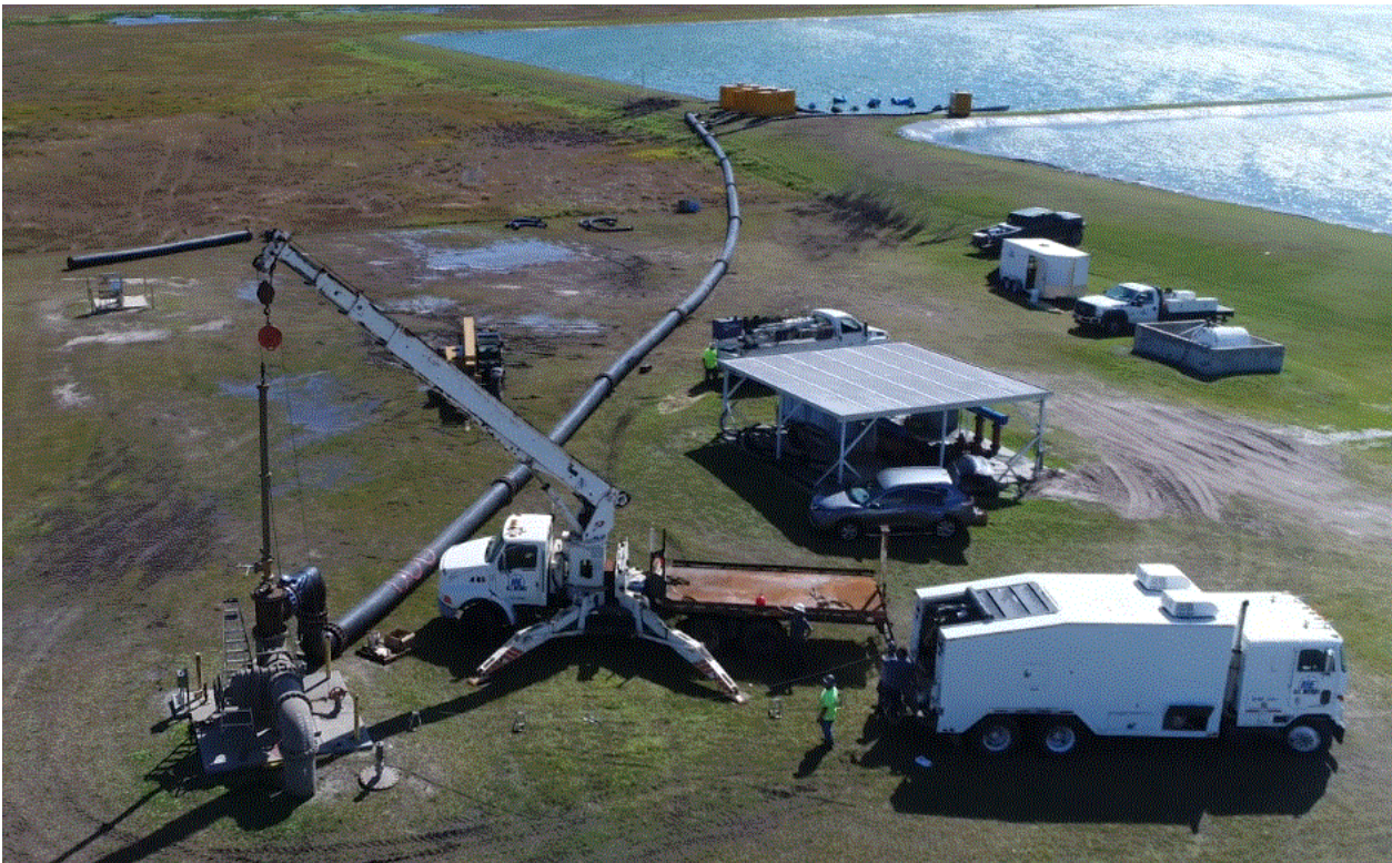
Photo 1. Photo showing the temporary pipeline leading from the lined temporary pumps (next to the lined pond) to the injection well in the foreground. The crane was used to hold the standpipe in place on top of the injection wellhead to allow the memory gauges to be installed to a depth of 2,750 feet bpl using the geophysical logging truck (white truck in the right foreground) logging wireline. Note: The photo shows 4 temporary pumps near the lined pond. One additional pump was brought to the site prior to beginning the test.
