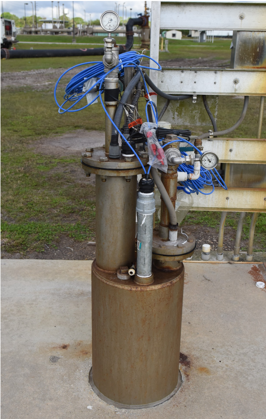
Photo 4. Photo showing primary and back-up In-Situ Level Troll 700 transducers installed in the upper and lower monitor zones of the dual-zone monitor well.
