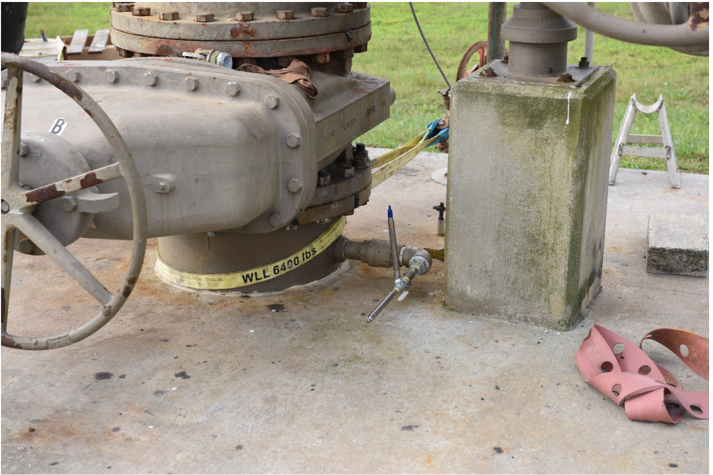
Photo 3. Photo of the primary and back-up In-Situ Level Troll 700 transducers (located in approximately the center of the photo) used to record injection wellhead pressures. The large 24-inch diameter gate valve remained open throughout the test so that the memory gauges could remain the well throughout the entire test. A temporary 18-inch diameter butterfly valve installed at the pipeline-wellhead connection was used to shut-in the well.
