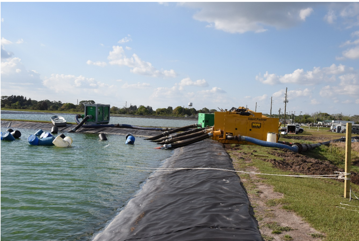
Photo 2. Photo showing the 5 temporary test pumps and pump intakes. Floats were used to keep the pumping intakes off the bottom of the lined pond.
